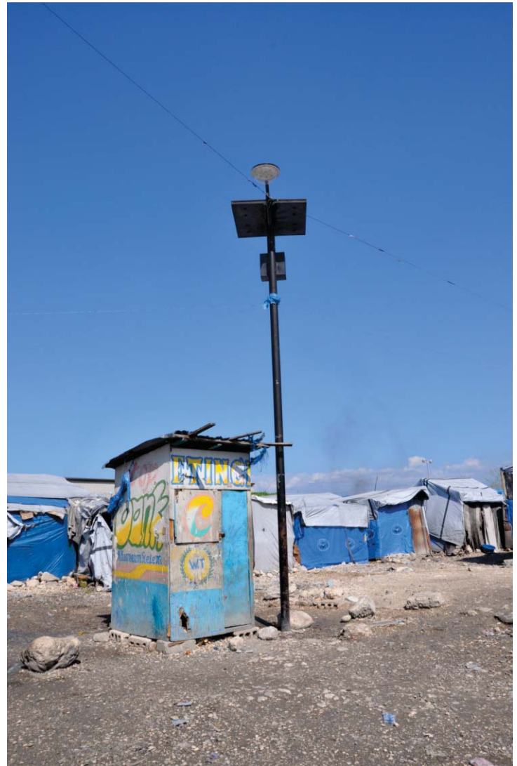
Adequate and strategic lighting was installed around public washroom.
