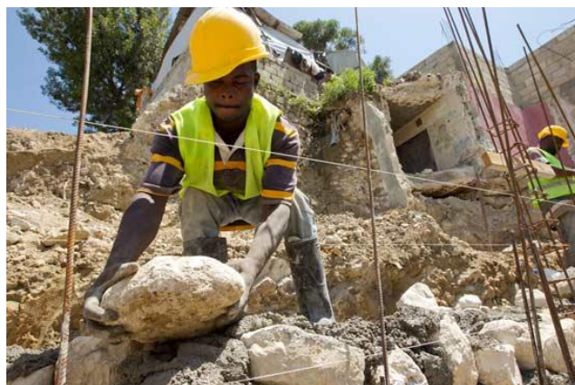
A Haitian worker undertakes rehabilitation and reconstruction works of neighborhoods affected by the earthquake. Credit Photo : MINUSTAH.
